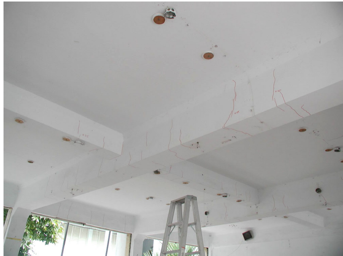
Fig. 11 Cracked beams after the vertical load test
