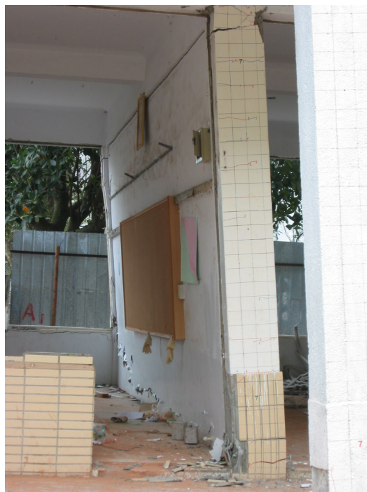
Fig. 15 Brick partition wall deflected in out-of-plane direction
